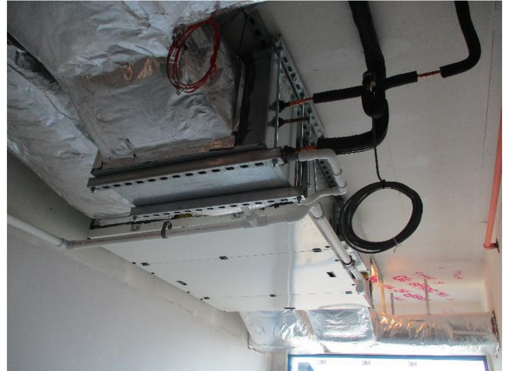
Post-tempered ventilation from ERV with DX heating/cooling
