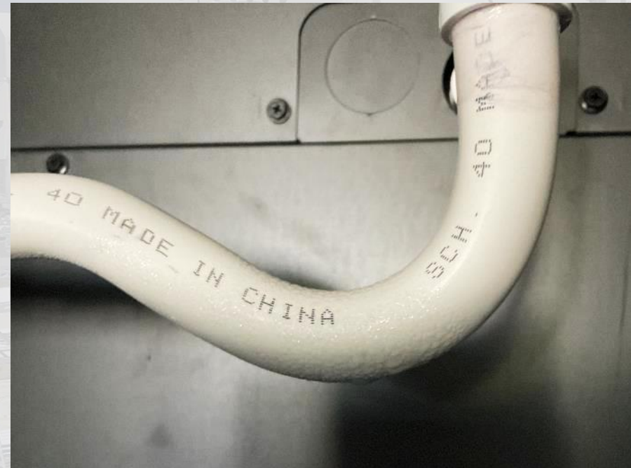
Condensation on plumbing
